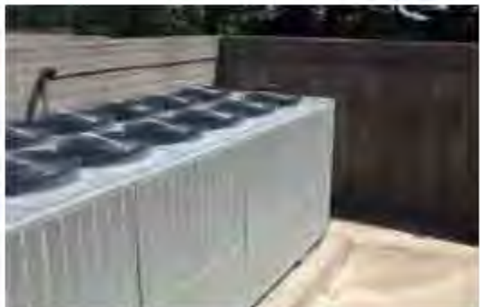
Chillers located north of Fine Arts building
